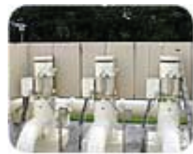
Sound panels installed at an industrial sewage pumping site to eliminate noise pollution to the surrounding park and residential areas.
